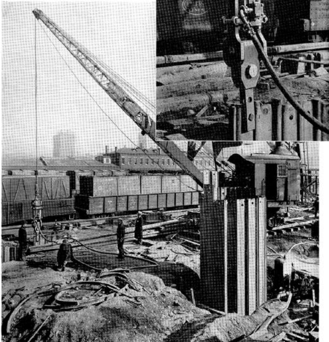
McKiernan-Terry No. E-2 Pile Extractor withdrawing heavy steel sheet piling which had been driven to a penetration of 75 feet and was bonded to concrete 35 feet on one side. The extractor, operated from the boom of a crane, completed the job without difficulty.
